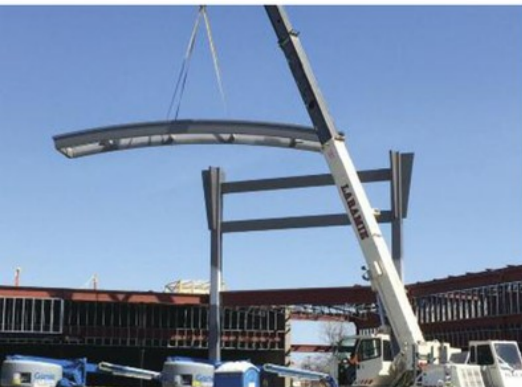
▲ Sign Monument steel erection showing two cranes lifting, one of three, field assembled, 9,000-lbs. rolled steel eyebrows.
