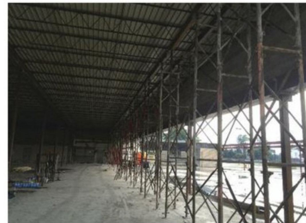
▲ Shoring was used to support the existing roof so that joists could be shortened and modified in the field.
